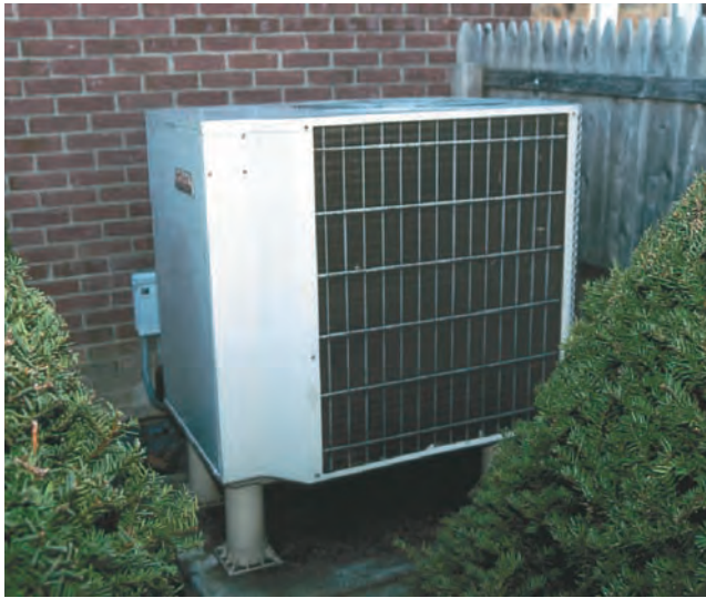
figure 11.11 The exterior heat-exchange coils for an air-to-air heat pump are usually located behind the house or building.
